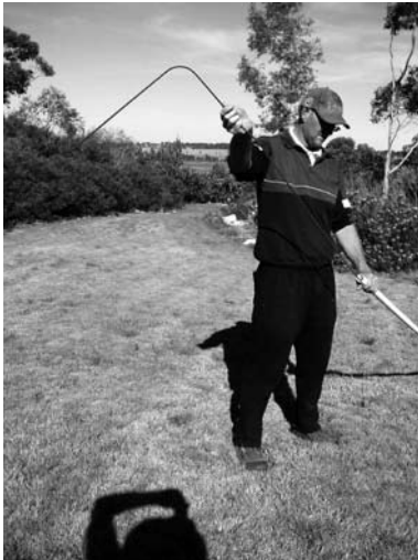
3) Feed the balance of the steel reinforcing about 3 meters into the pipe.
